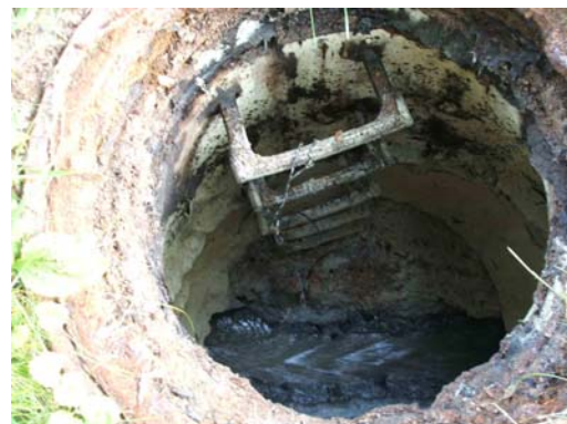
Manhole as sulphur factory
